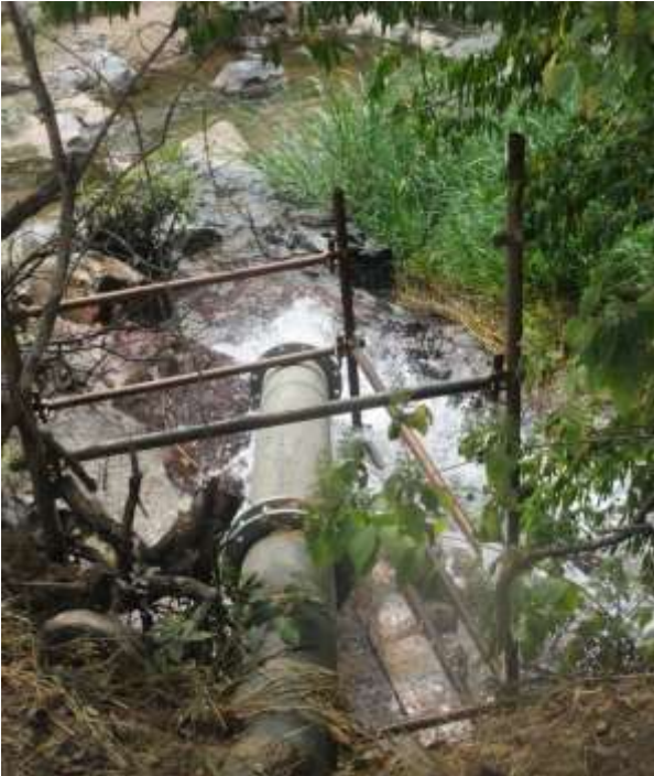
Discharge from the Sere River to the Mine's treatment Plant
