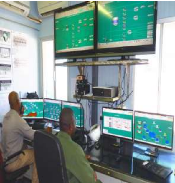
Control Room of the on-site water treatment plant
