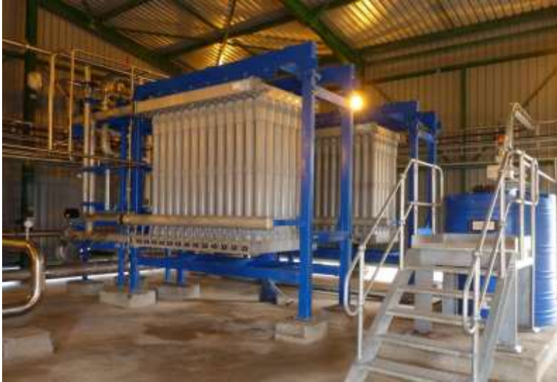
FIGURE 9 REVERSE OSMOSIS WATER TREATMENT PLANT IN KARONGA
